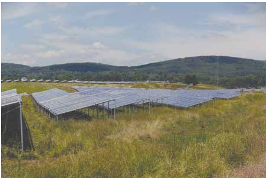
A fifteen-megawatt solar array at Fort Detrick, Maryland
