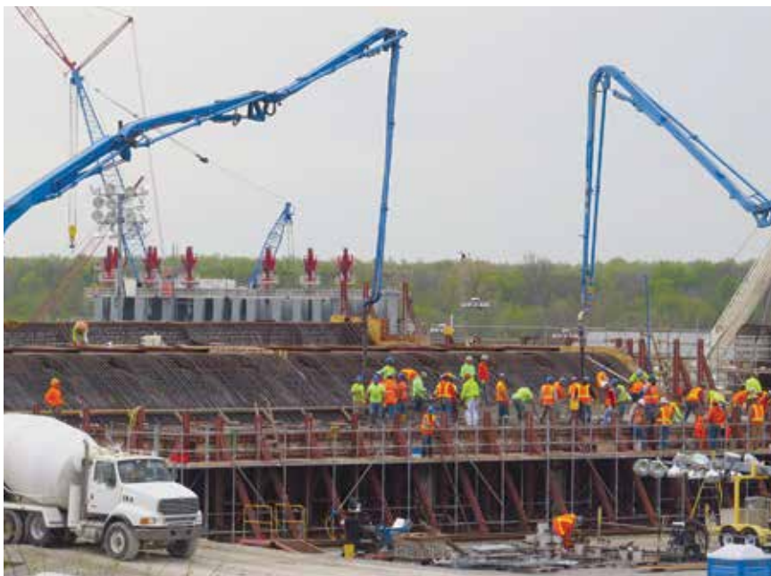
Olmsted Locks and Dam conducts a concrete placement on its eighth navigable pass shell.
