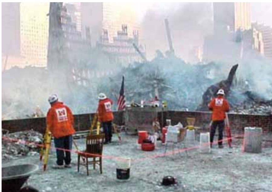
A survey team from the Corps of Engineers assists in checking the integrity of structures following the 11 September 2001 attack in New York City.
